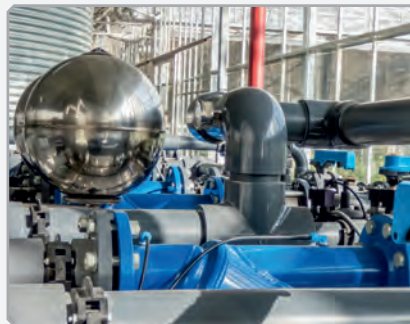
Industrial Process Lines
